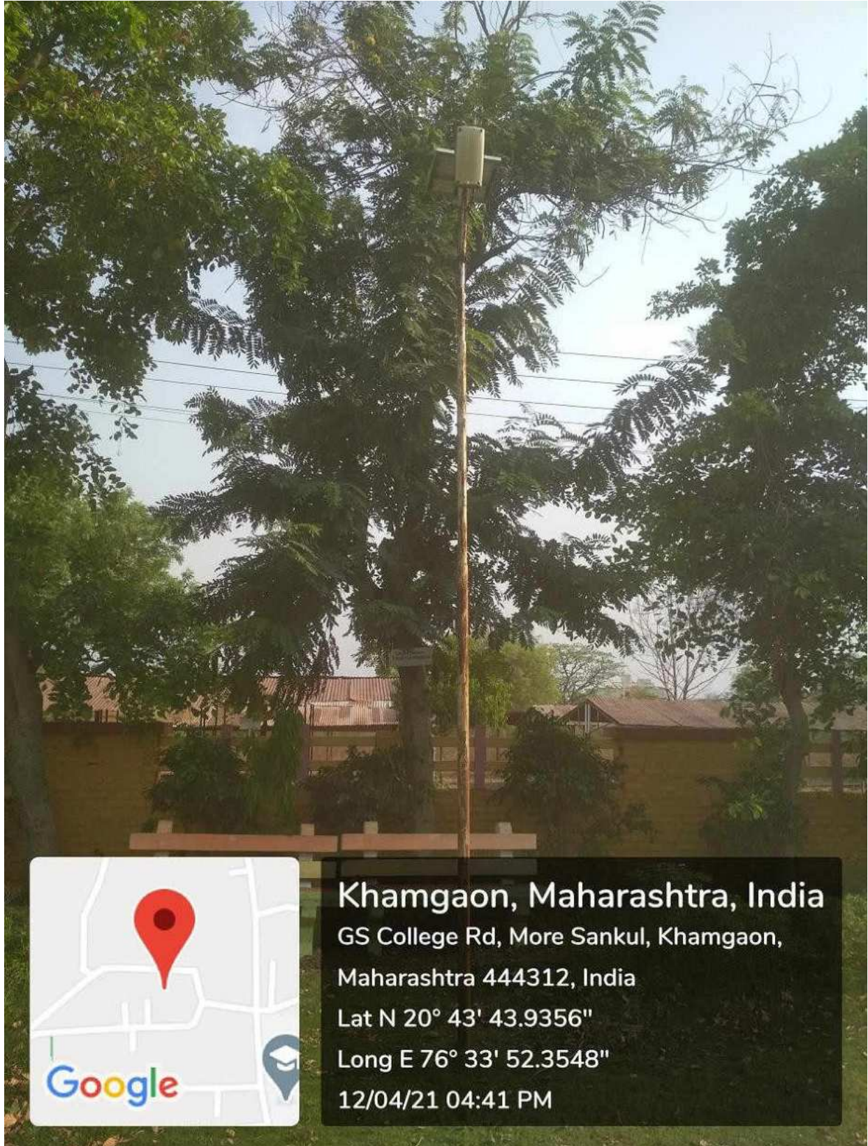
Photo 2: Solar street lamp
