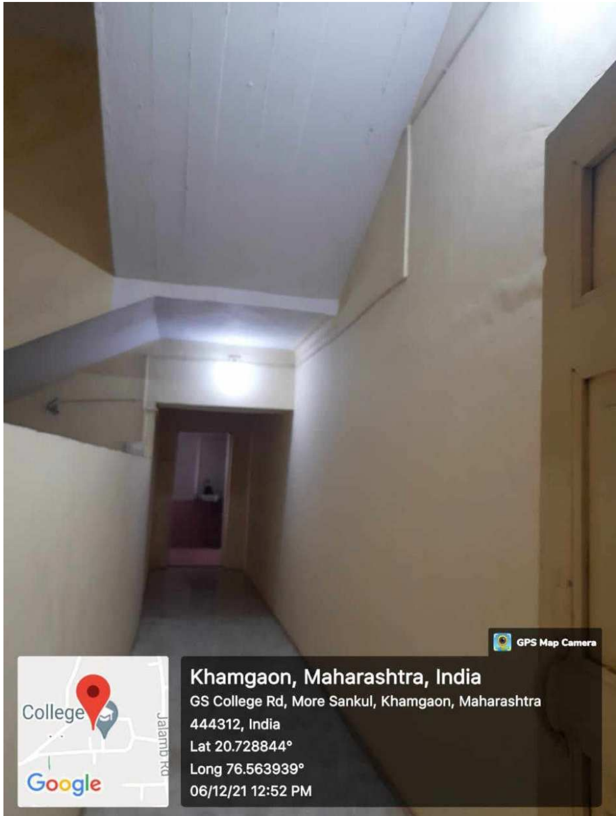
Photo 4: Sensor based light installed in the paassage
