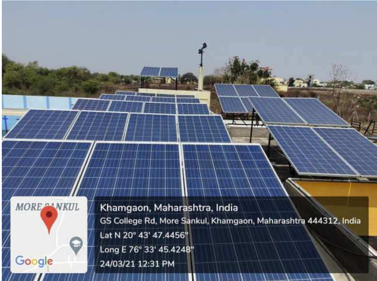
Photo 3: Solar Panels installed on the Swimming Pool
