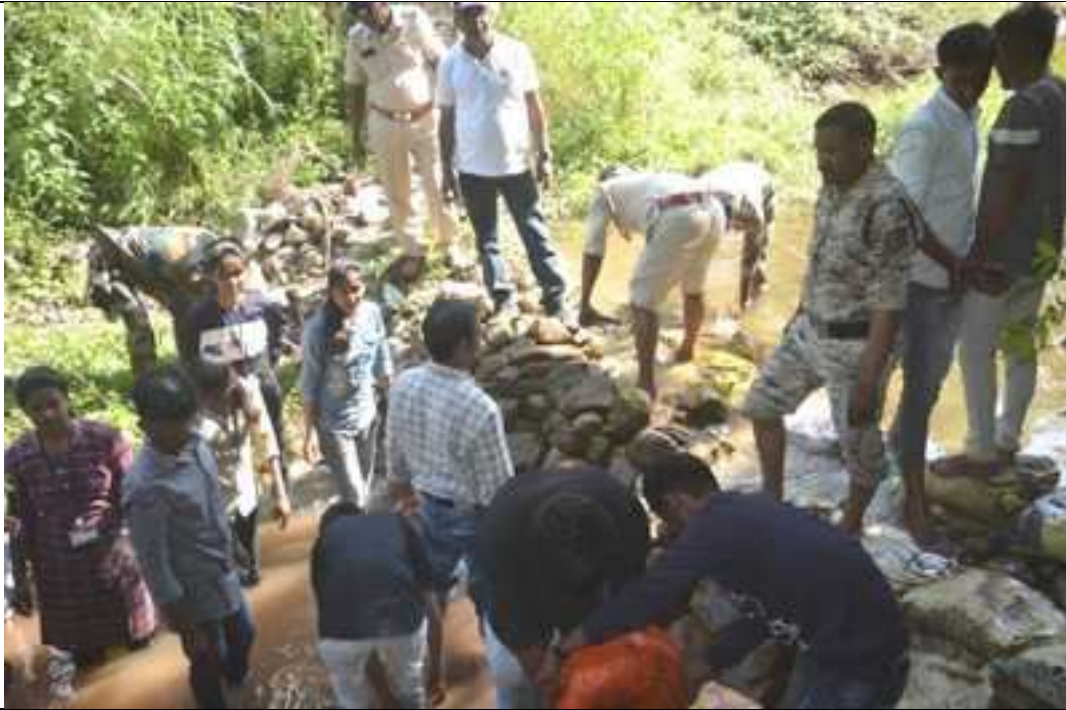
Dr G.B.Kale students and forest staff - Bandh Construction at Nakshatra Ban ,The Dnyanganga Wildlife Sanctuary
