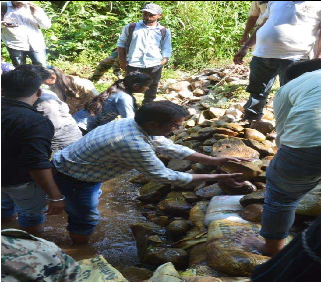
Dr G.B.Kale students and forest staff -Bandh Construction at Nakshatra Ban, The Dnyanganga Wildlife Sanctuary
